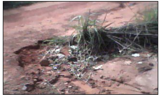
Fig 2.1: Gully Unit a (Agulu Uwani Road)
