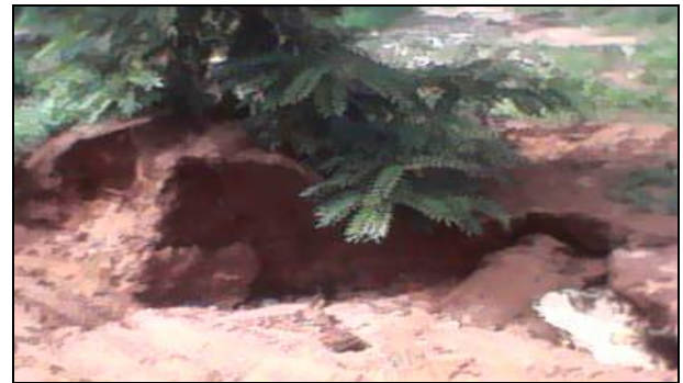
Fig 2.2: Gully Unit B (Enuguodousu Road)
